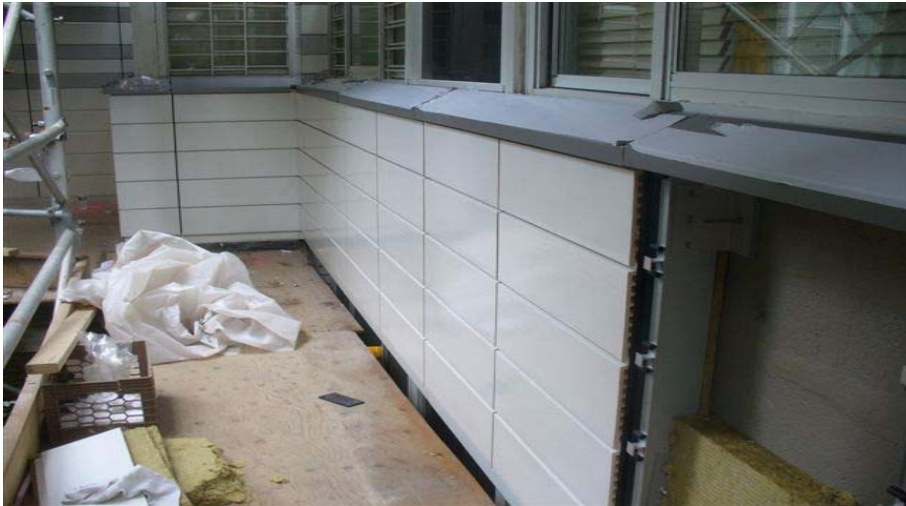
Photos shows tiles inserted with sills in place and showing part insulation
