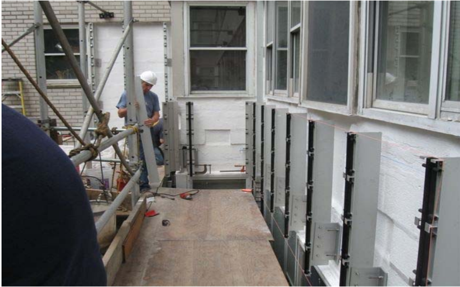
Photo shows run of vertical tracks set at correct levels and positions
